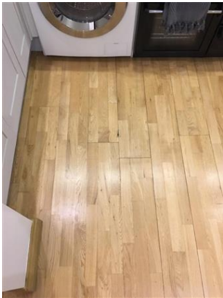
Flooring to match living room Laminated parquet oak effect Scuffs and marks Wear and tear Clean
