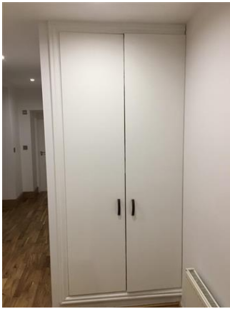
Walk-in Storage Exterior door Doors painted white with leather door handles Interior Doors with fire rated panels Damaged in the handles level
