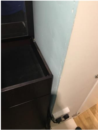
Crack on the wall
