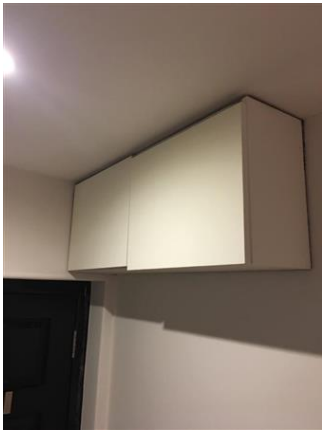
Fuse box cabinet Painted white
