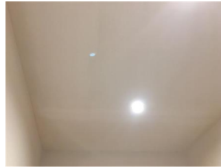
Under paint defect Crack
