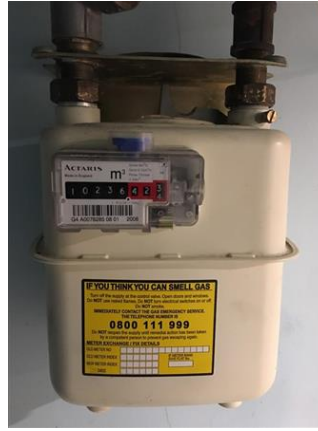
Gas meter G4 A0078285 08 01 Meter readings 10236 424
