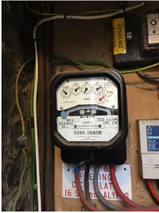
Electricity meter S58A06608 Electricity readings 88582
