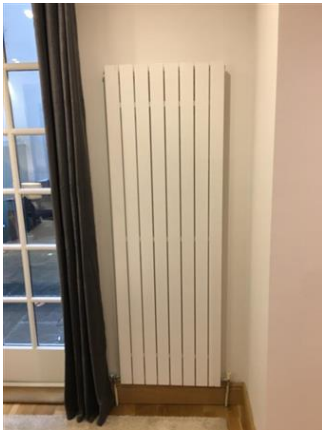
Vertical radiator painted white
