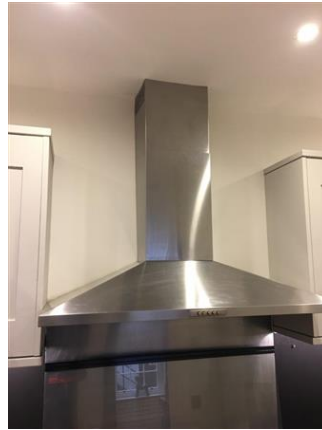
stained steel, triple mesh, with lighting and diffuser Wear and tear Clean
