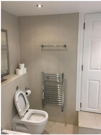
Walls grey tiles Wear and tear
