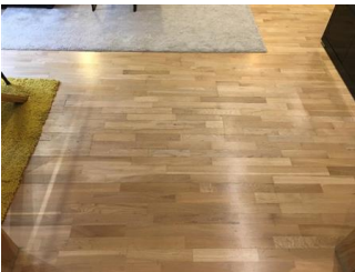
Flooring to match hallway Laminated parquet oak effect Scuffs and marks Wear and tear
