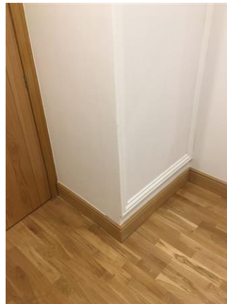
Cracks in places Medium size dent painted over behind the door. Handle level
